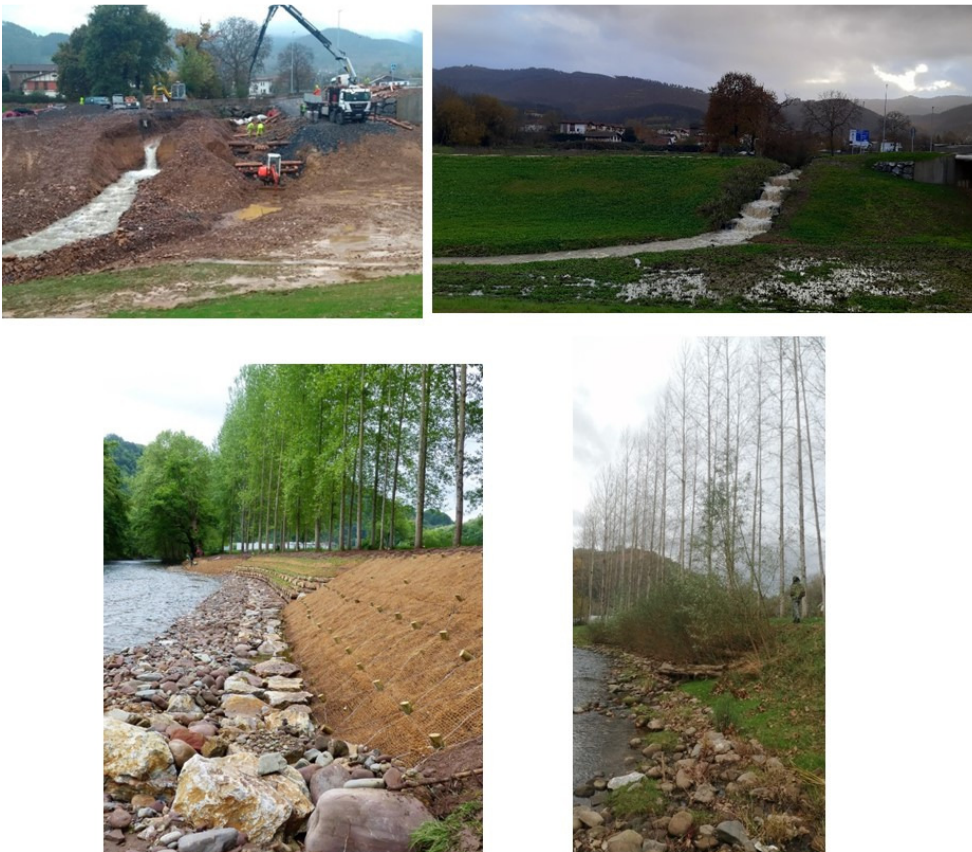
Fig. 1. Examples of successful soil and water bioengineering (SWB) works in the Mediterranean. A) the restoration of the Sollano Stream, (Zallain, Spain) by Sangalli Coronel y Asociados S.L – URAGENTZIA (top photos). B) Stabilization of a stream bank in Rio Baztan (Navarra, Spain) by Sangalli Coronel y Asociados S.L – GANASA (bottom photos).
